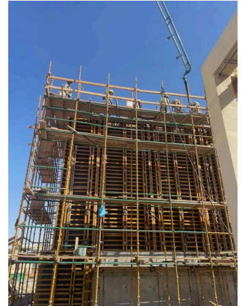
Laborers working safely on scaffoldings during the pouring of the reservoir wall - September 11, 2023. Photo credit: CDM International Inc.
