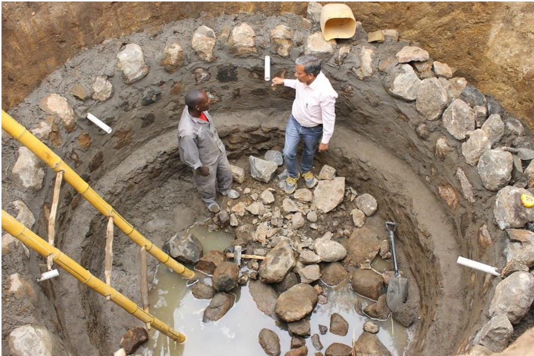
The pipes allow for seepage water to enter the well from the sides.
